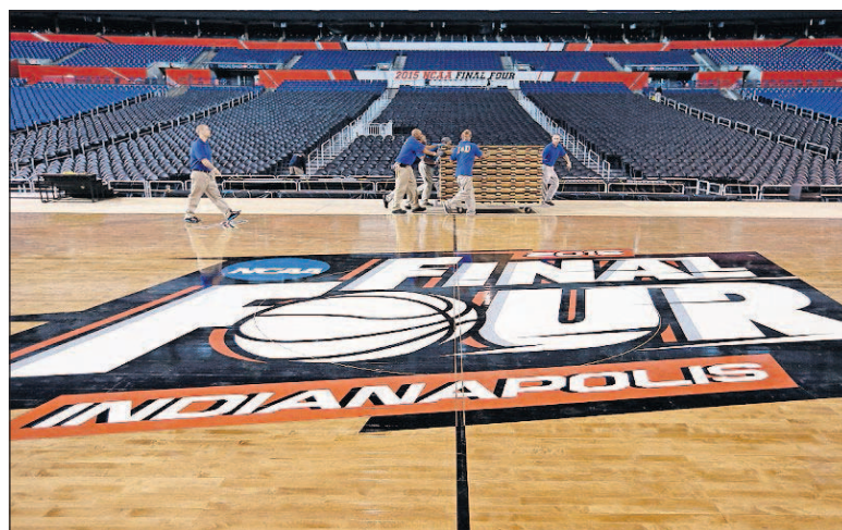
Workers at Lucas Oil Stadium install the court in Indianapolis as they prepare to host the men's NCAA Final Four games on April 4th and 6th. NCAA officials say they are troubled by the new law in Indiana that critics fear could permit discrimination against gays and lesbians, and they "will assess all our championships in the state of Indiana," including next year's women's Final Four. THE ASSOCIATED PRESS
